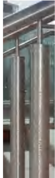
Rusting of iron contamination during the service life of stainless steel is unsightly. Removal can be time-consuming and expensive.
